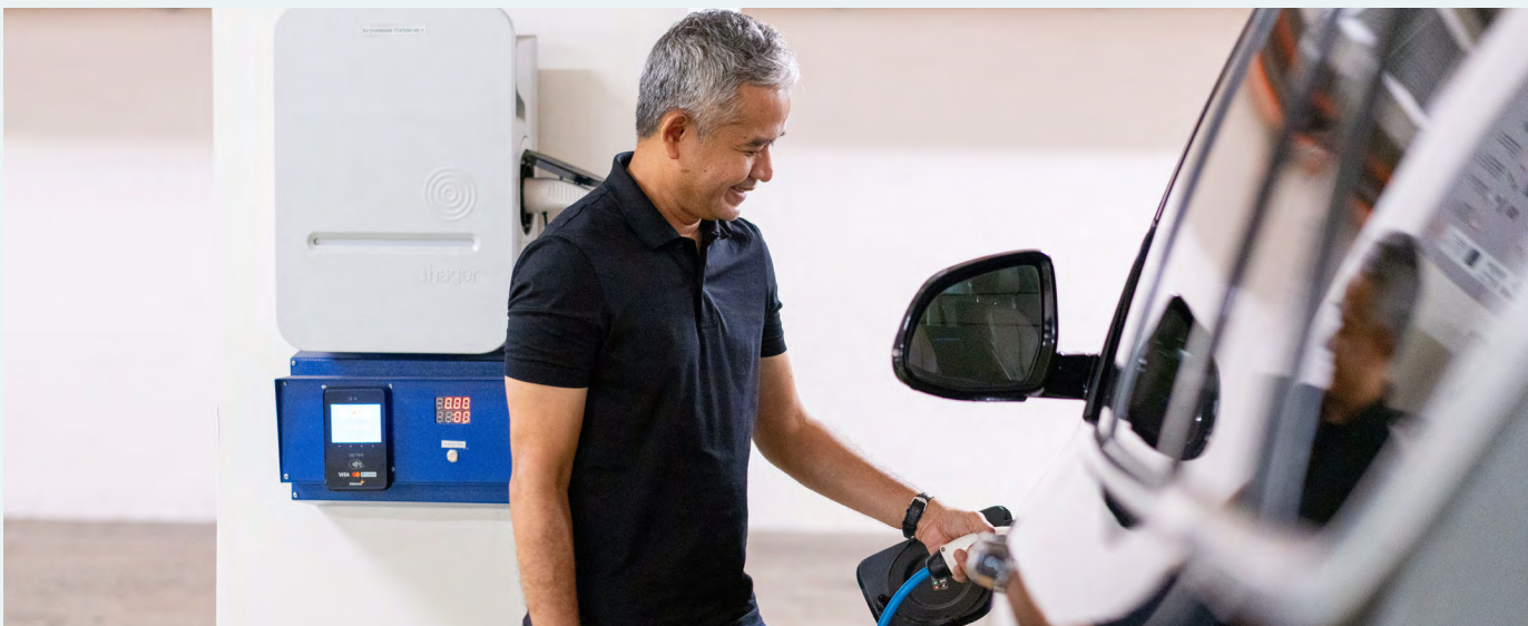
Electric vehicle (EV) charging stations at Residensi Solaris Parq showcasing our commitment to reducing carbon emissions
